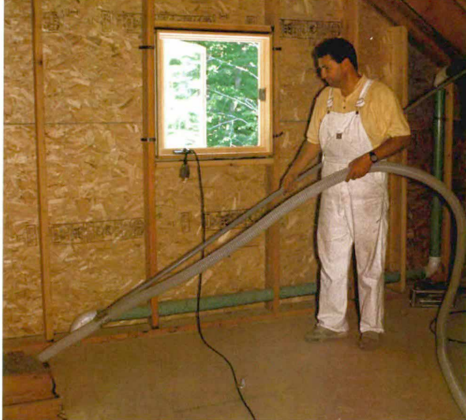
A guide rod supports the hose. Simply 1-in. conduit duct-taped to the hose end, guide rods can be joined together to coax floppy hoses deep into building cavities.
